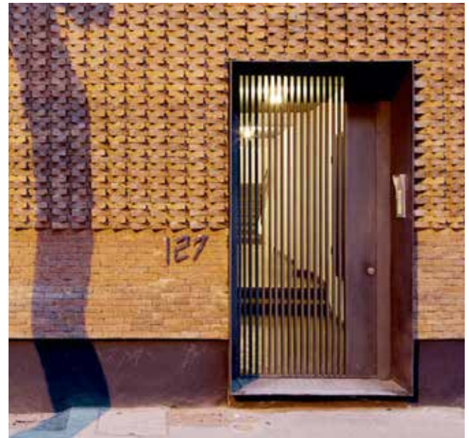
Alternate courses of stretcher bond angles at 30° from the direction of the brickwork.
